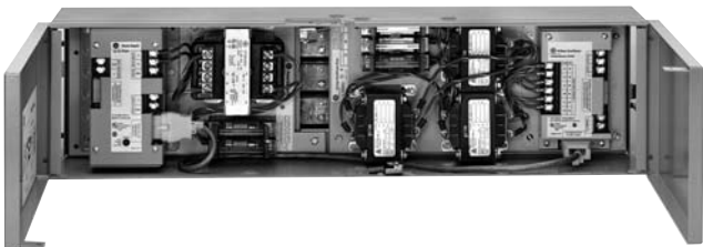
Voltage Module Interior View
